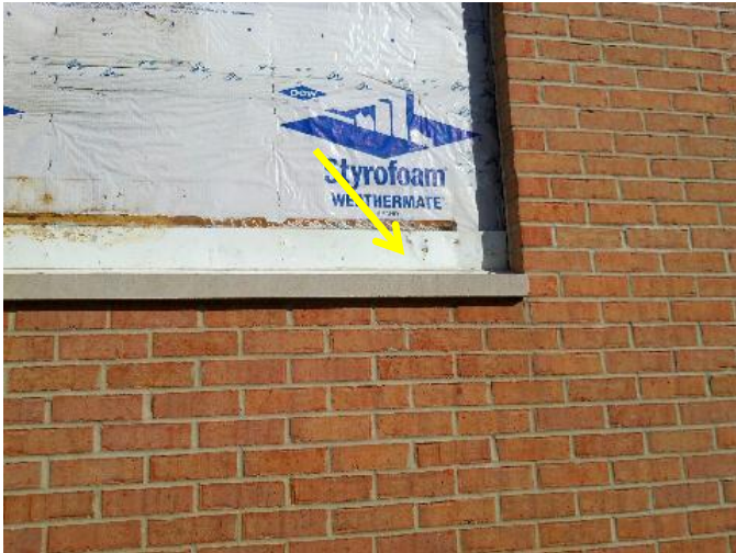
Typical flashing installed between the panels and brick. Note the flashing is installed on top of the building wrap. The flashing needs to be installed behind the building wrap and the top edge of the flashing needs to be sealed to the wall sheathing in order to be effective.
