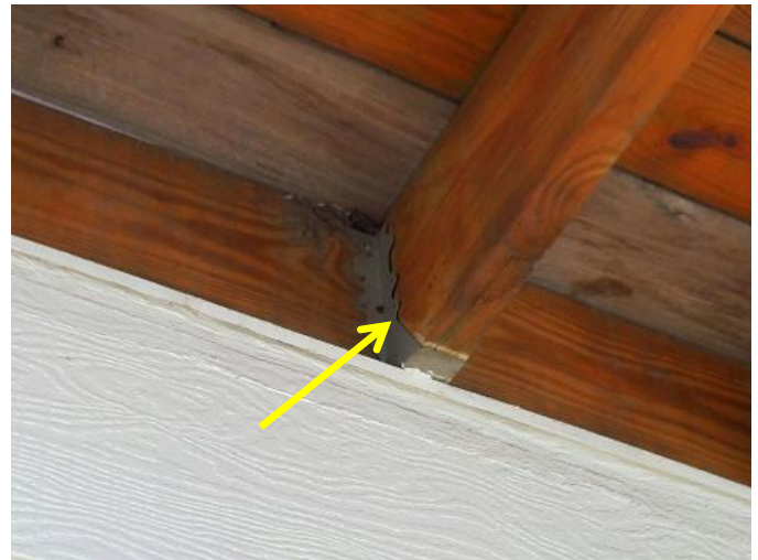
Several of the joist hangers did not have nails installed between the joist hanger and joist. The joists cannot be properly tied to the ledger board without fasteners installed in all joist hanger holes.
