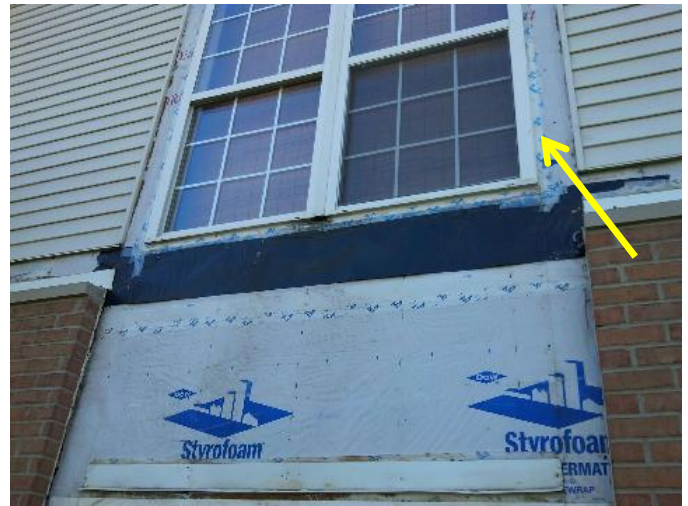
Note the Tyvek tape installed around the perimeter of the windows which is not an acceptable method of window flashing.
