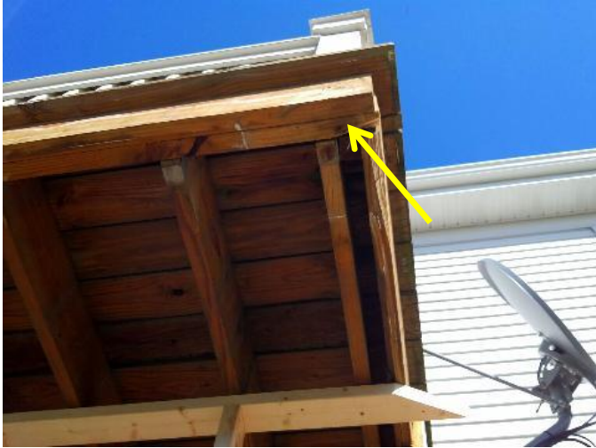
View of the double rim joist and single outside joist. The existing 4x4 columns were noted to be toe-nailed into the bottom which is not the proper way to attach a column to the deck framing.
