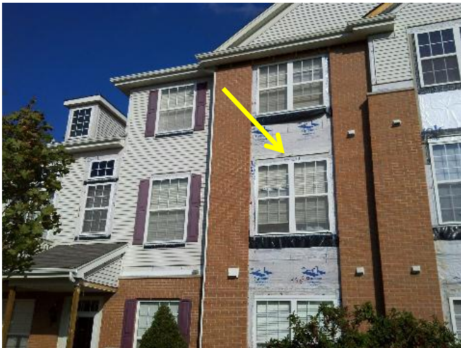
View of the locations at the building that panel siding is installed between the windows. Note the z-flashing installed at the top of trim boards but the flashing is installed on top of the building wrap in lieu of behind the building wrap.
