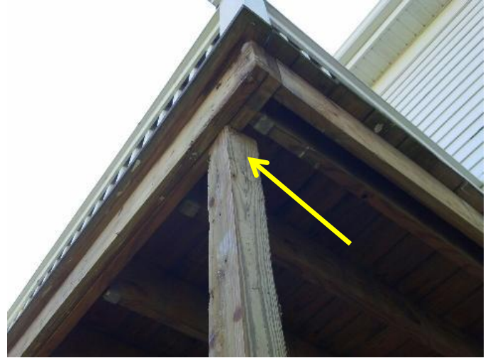
View of existing 4x4 column in place prior to removal. Note the column is only in contact with the inside member of the double 2x8 rim joist. This creates an unstable deck condition.
